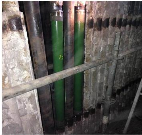
Figure 4. Tubes in the steam reheater (2014)
