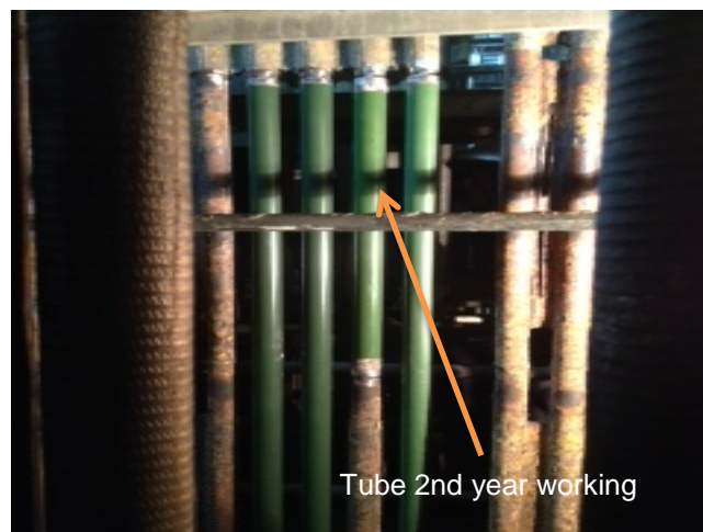
Figure 7. Tubes working in Urban Garbage Power plant. Installed 27 th April 2015
