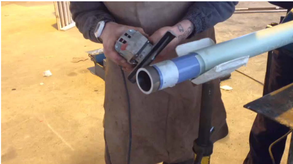
inside or outside the boiler
