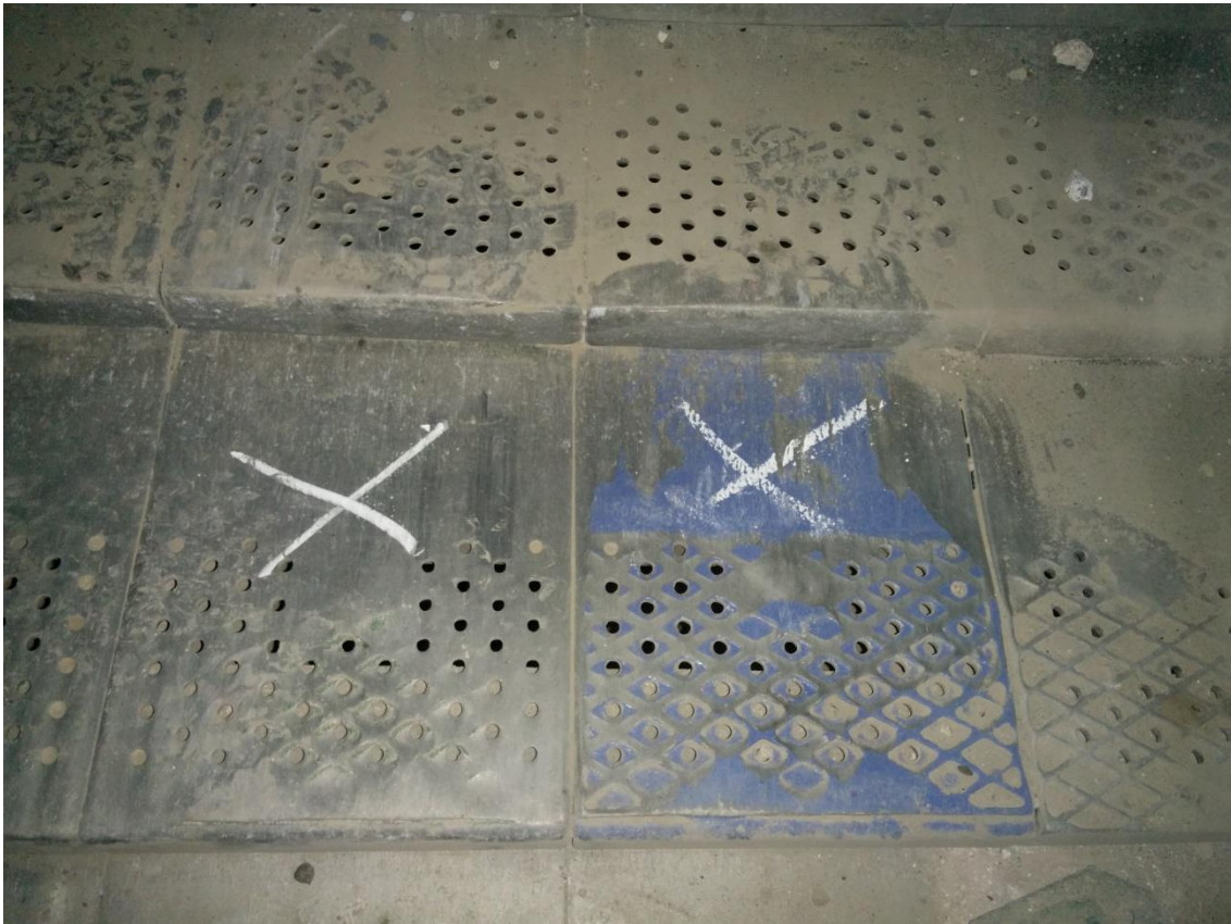
Both plates after just one year of continuous operation.
