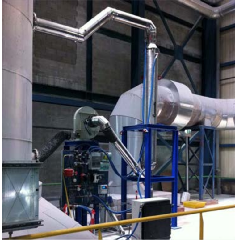
200 KW CONDENSER on first trials AFTER filters.... Prior of being installed... BEFORE FILTERS
