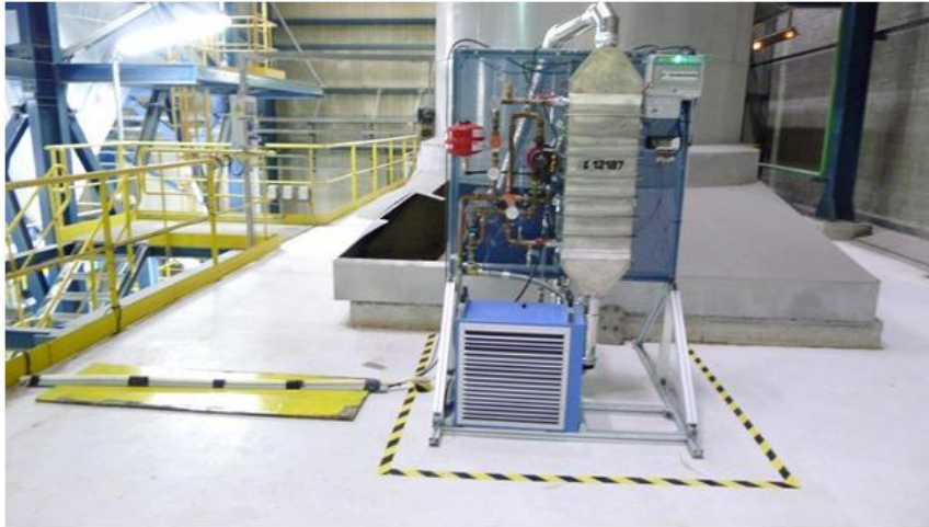
Figure 1. 5kW fume condenser prototype at a Urban Waste Power Plant
